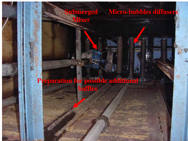
Figure 2.7. Micro-bubbles diffusers and submerged mixer
