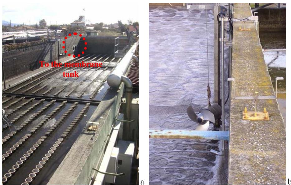
Figure 8.7 a-b. Aerators (a) and mixers (b) in the AC tank
